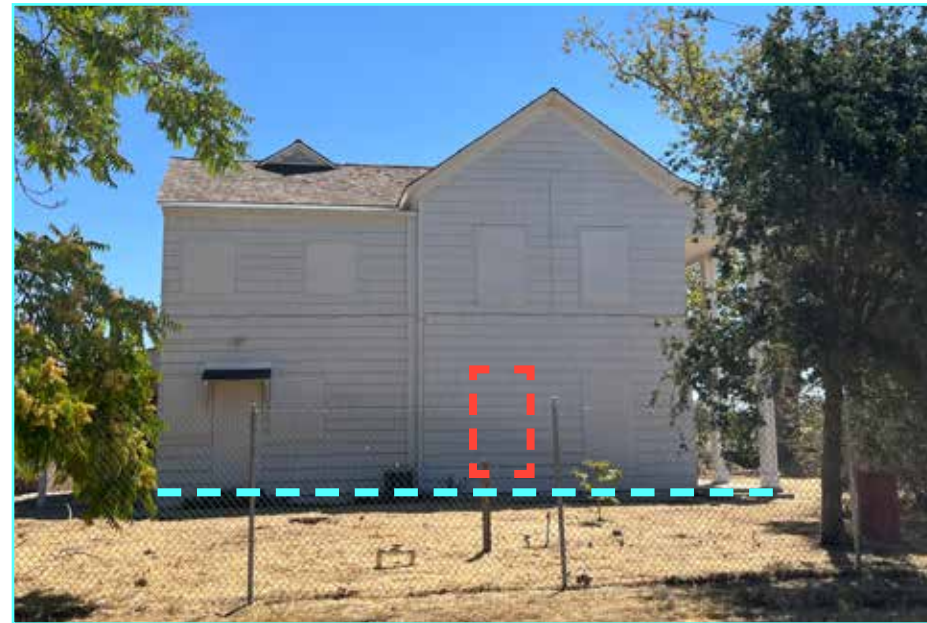
Figure 15: The west elevation of the Main House, view east (2024). The location of a window recommended to be reopened is outlined with a dotted red line. The approximate location of a new raised deck is indicated by light blue dashed line.
