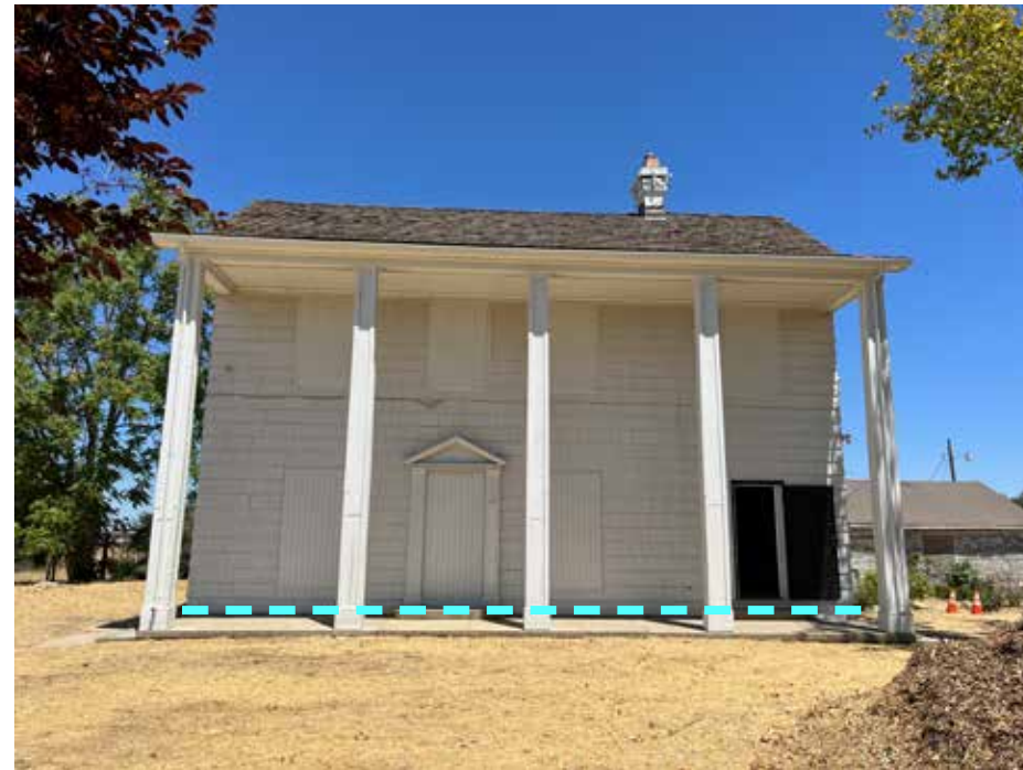
Figure 12: The front (south) facade of the Main House, view north (2024). Approximate location of new raised deck indicated by light blue dashed line.
